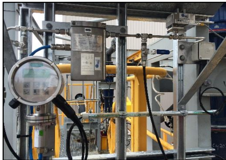
The neat installation of the Siemens Coriolis flow tube, transmitter and the Hanbay actuator completed by The process plants own E/I department.
